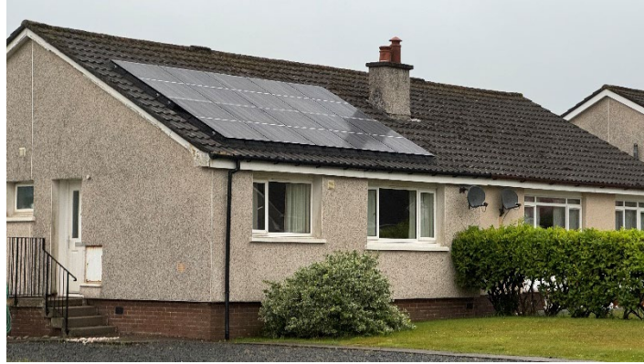
Figure 13: Residential installation of Solar PV and battery system.
