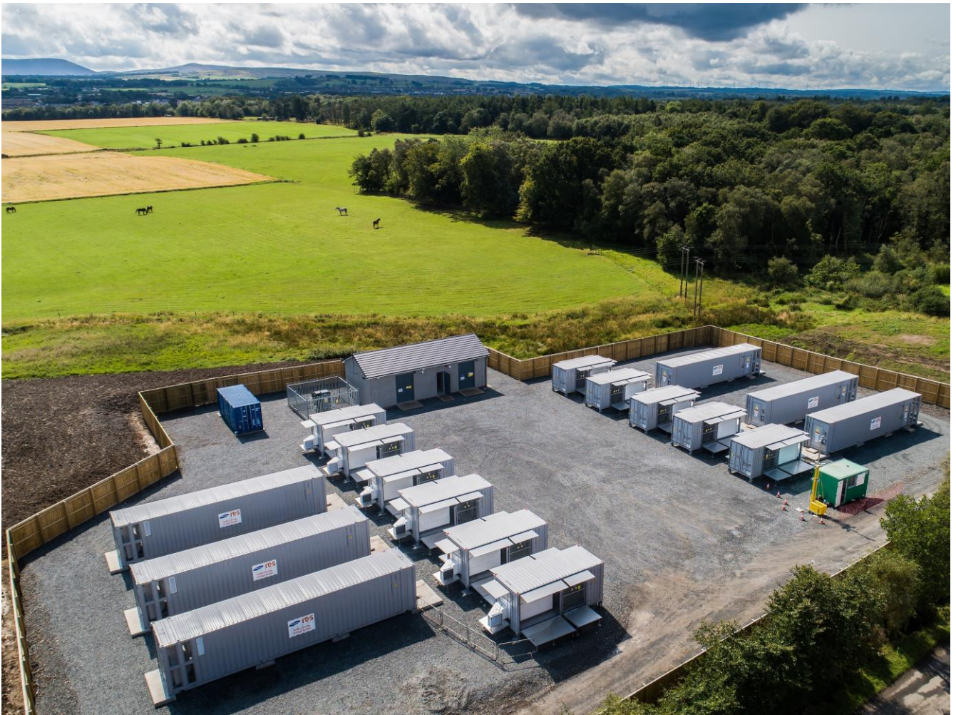
Figure 3: Broxburn 20 MW battery storage project, West Lothian, constructed in 2018 to provide sub-second balancing services to National Grid (image RES Ltd/Keith Arkins)
