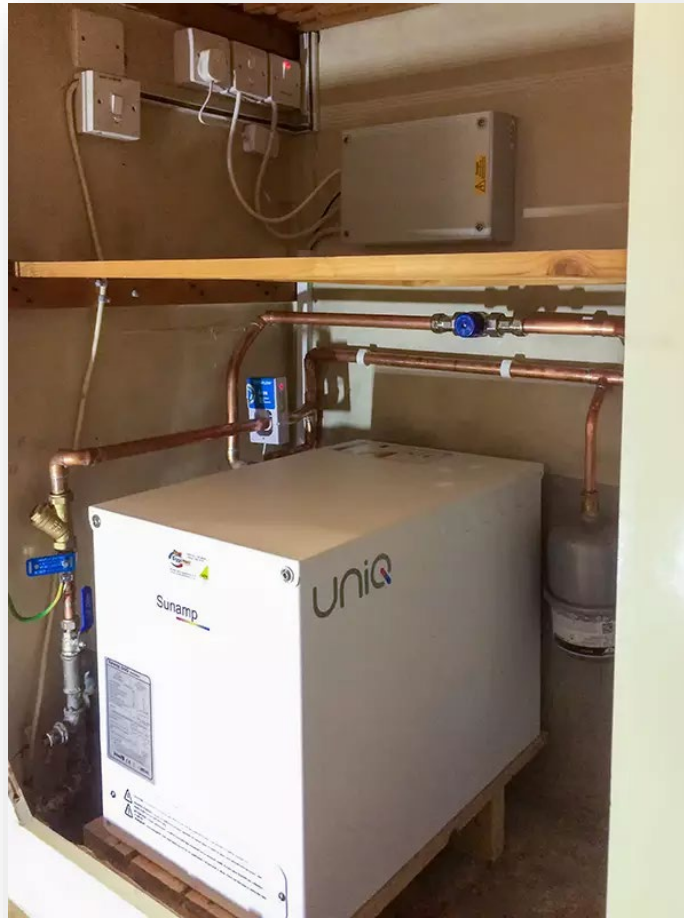
Figure 1: In-situ Sunamp UniQ heat battery 20
